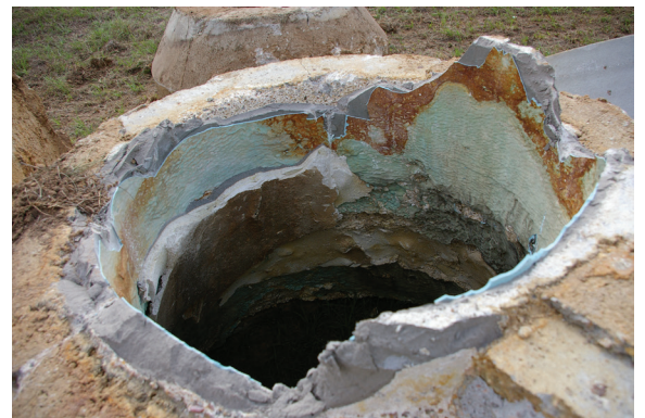
☐ MULTIPLE LAYERS OF FAILED REHAB COATINGS
