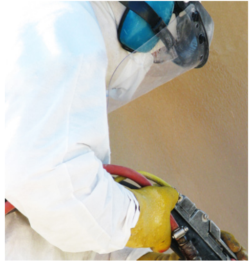
The tank surface is abraded to allow for a strong mechanical bond.
